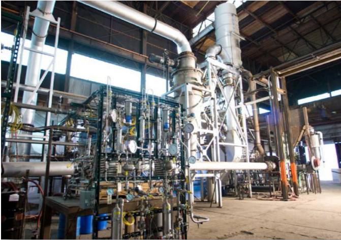
Hammond, Indiana 15 MWth Test Facility
